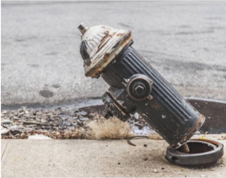
AI Detected Asset Type: fire hydrant at 95% confidence
