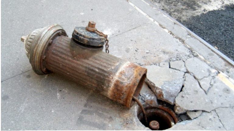
AI Detected Asset Type: fire hydrant at 95% confidence
